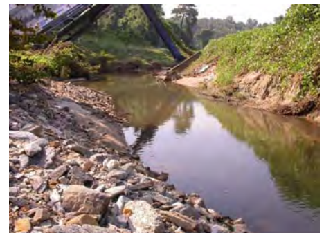
EXHIBIT 7 Channel Erosion: Contributes to Habitat Degradation and Sedimentation Problems in Beaver Creek
